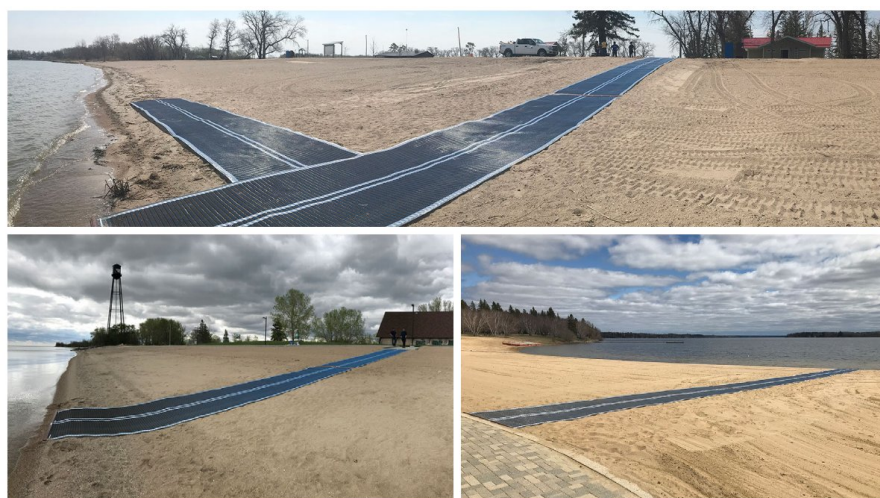
Three images of the Mobi-mats installed in provincial parks across Manitoba that provide a firm surface from the beach into water for people with mobility disabilities.
